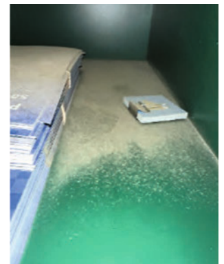
Mould in the storage areas of a police station front counter.
