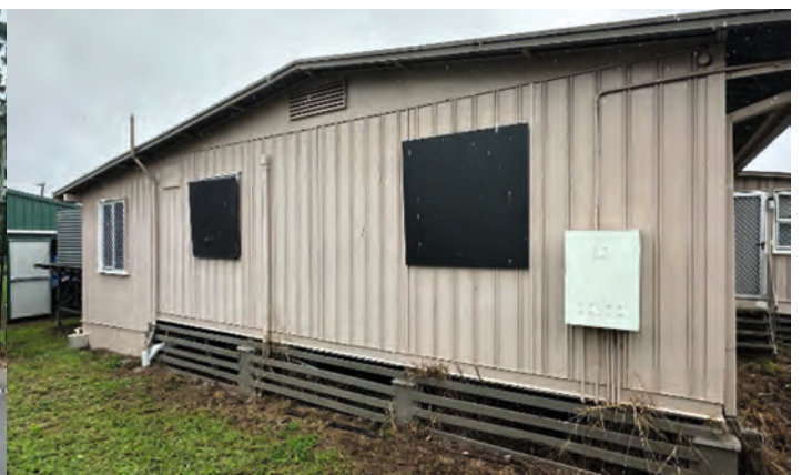
Police housing at Murgon where windows are boarded up due to offenders constantly smashing the glass.
